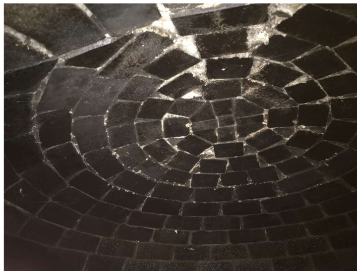
Efflorescence Stalactites from joints of dome
